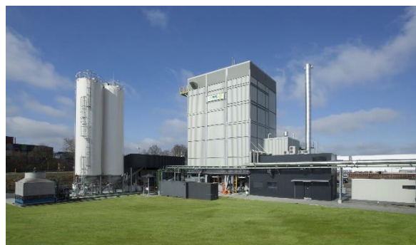
Figure 29: The Empyro pyrolysis plant in Hengelo, The Netherlands
